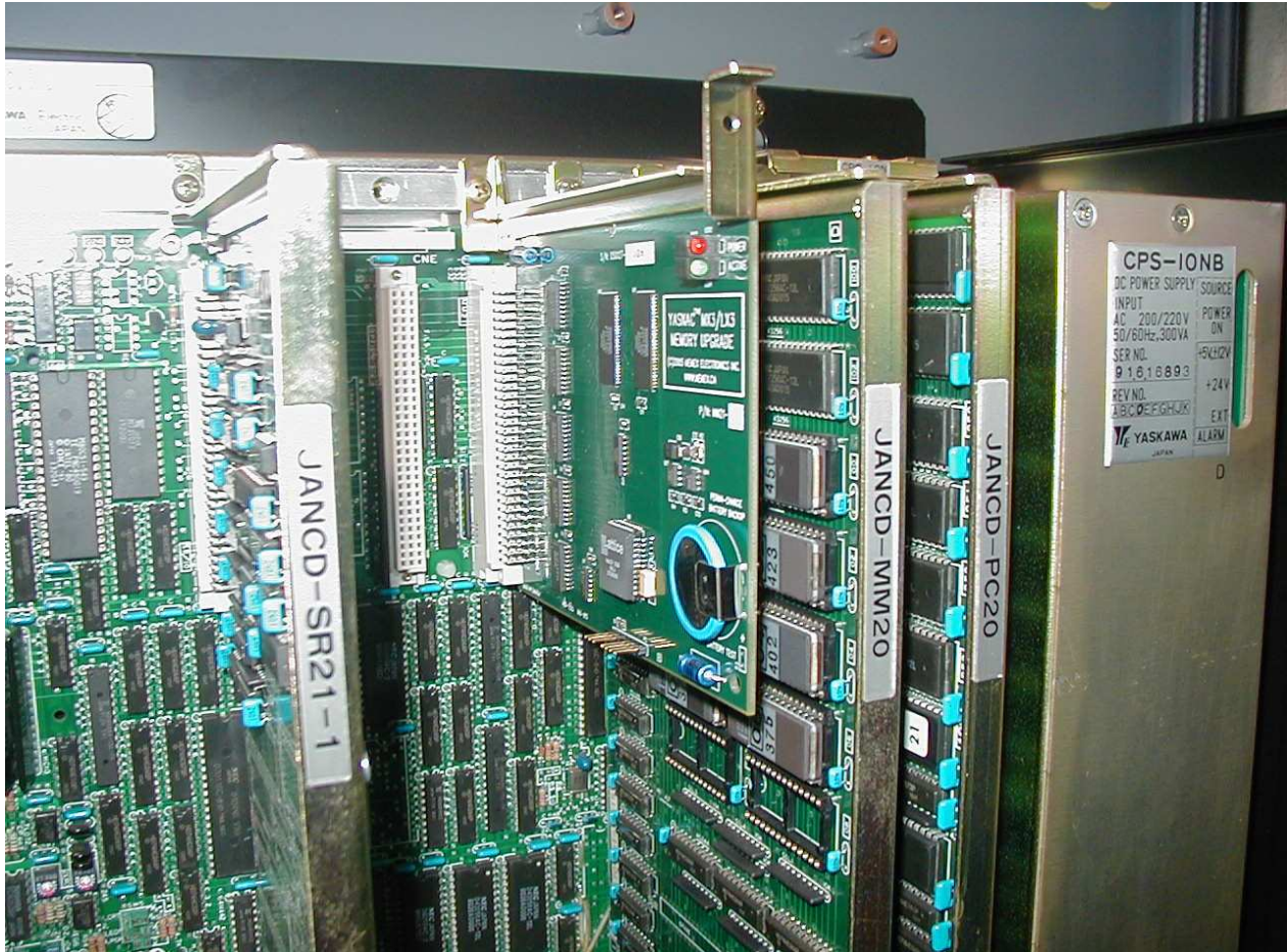
An installed Memex MX3 Board in the MM21 slot beside the MM20 Board.
