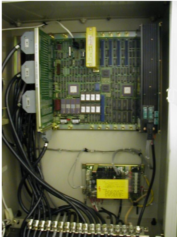
Fanuc 10A – all upgraded (no empty sockets)
