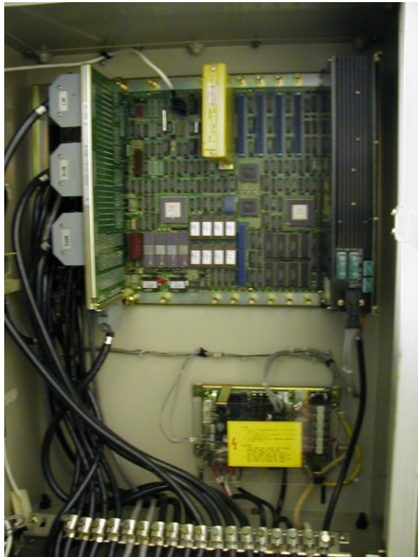
Fanuc 10A – all upgraded (no empty sockets)
